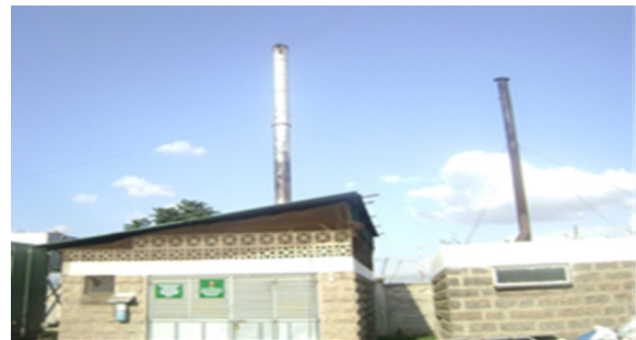
Plate 1: New and old incinerators at the Hospital
