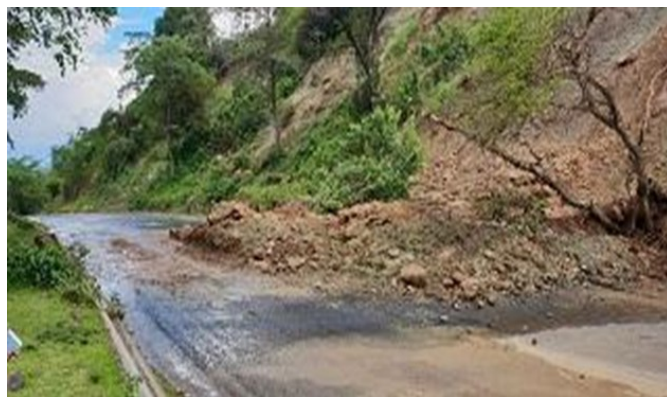
Plate 2: Landslide along Iten-Kabarnet Road (Source: KeNHA, 2018)
