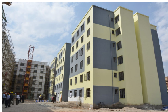
FIGURE 1 Ongoing construction work at Park Road Housing Project in Ngara estate, Nairobi Source: Authors 2020
