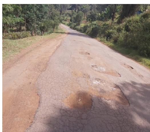
b) Cracks, pot holes and no drains at km 3.5
