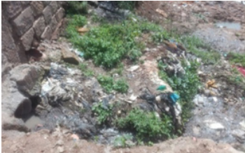
FIGURE 13 Sewer draining into Mathare River in Mathare North Informal Settlement Source: Field survey, 2025
