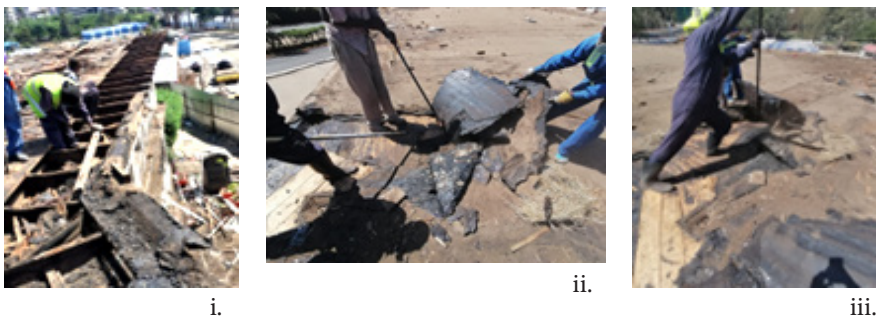
FIGURE 7c Flat roof demolition (i. Soffit, fascia and roofing joists removal. ii & iii. Stripping of the bitumen layer off the roof) Source: Authors 2020
