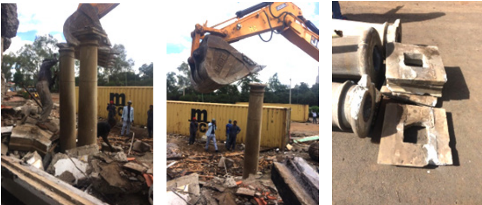
FIGURE 10b Precast column extraction and assessment of the degree of damage Source: Authors 2021
