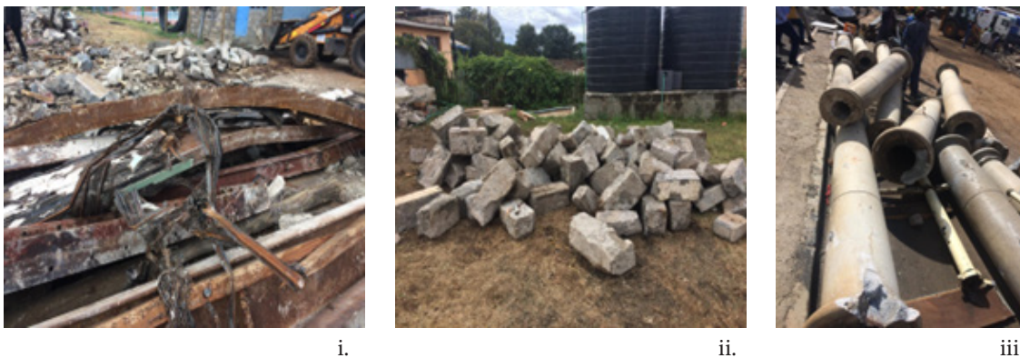
FIGURE 7e Material sorting and collection (i. Cast iron beams. ii. Salvaged Nairobi blue stones. iii. Stacked classical columns) Source: Authors 2020
